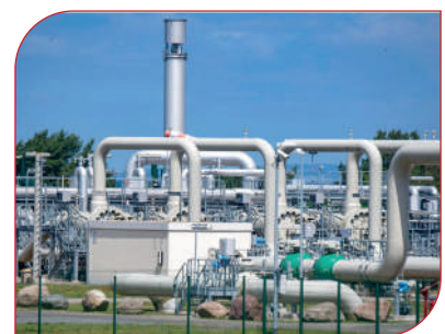
Gas Gathering Station Shahdol, Madhya Pradesh
