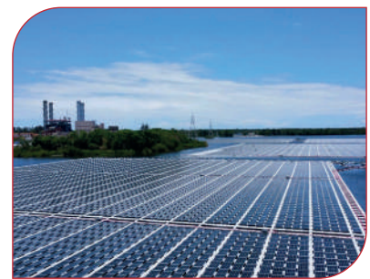
NTPC Floating Solar Power Plant Kayamkulam, Kerala
